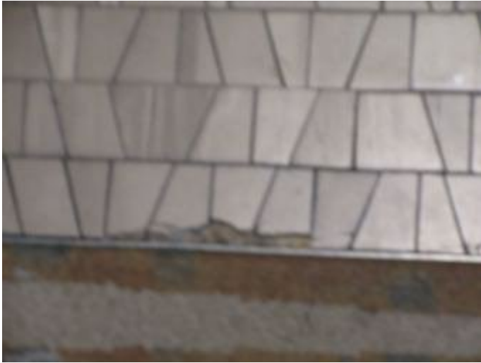
Deterioration of floor tiles at the Westin
