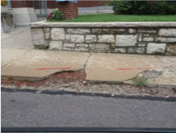
Deteriorated street improvements along Gillham.
